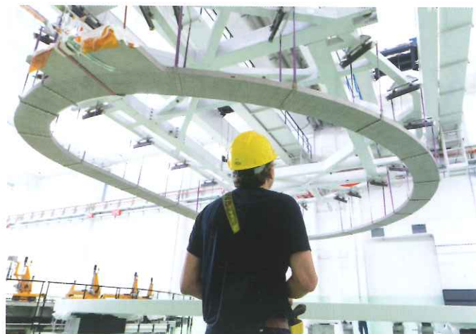
Technician lifting a Double Pancake to position it on another station, ASG Superconductors, La Spezia (Italy) © Andrea Botto
